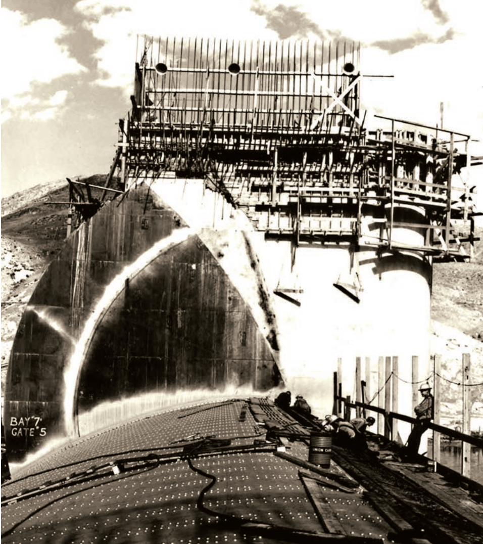
DRUM GATE IN LOWERED POSITION AT GRAND COULEE DAM. MAY 20, 1941. GIVEN THE DATE, IT IS POSSIBLE THAT WOODY WAS THERE THIS VERY DAY.
